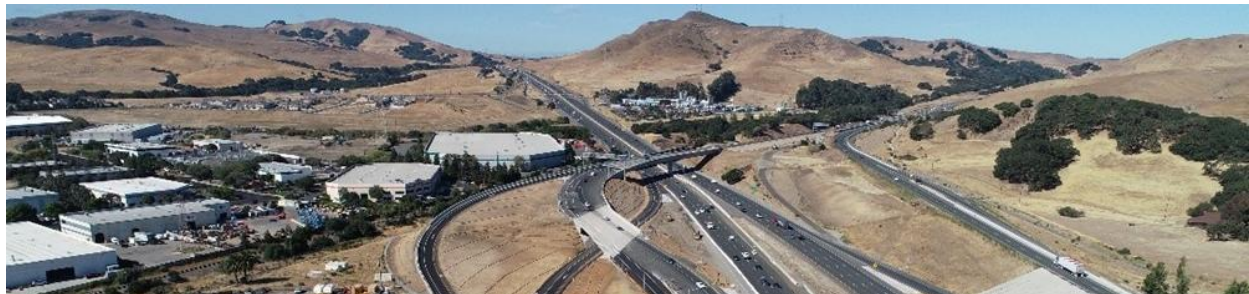
First RM3-funded construction package for the I-80/I-680/SR 12 interchange in Fairfield. Photo: Caltrans
