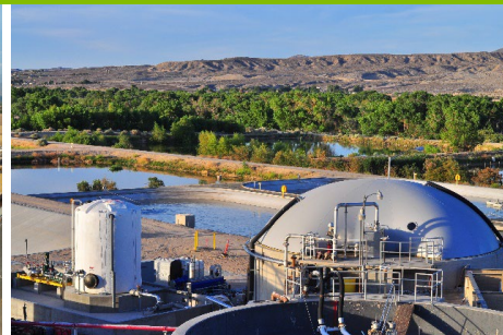
VICTOR VALLEY WATER RECLAMATION AUTHORITY VICTORVILLE, CA DBOOF
