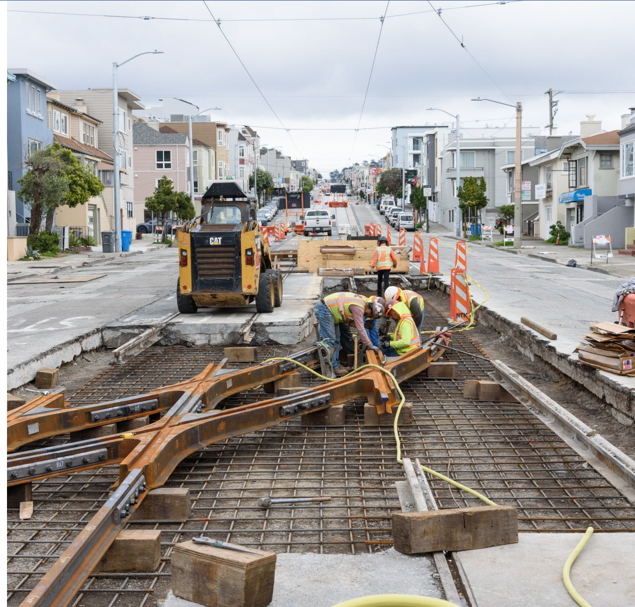
Photo Credit: SFMTA, San Francisco L Taraval Track Switches, 2024
