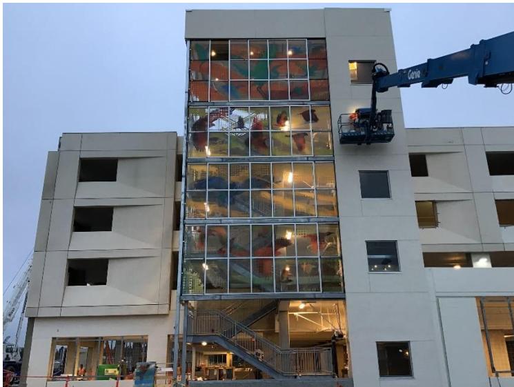
Photo of Dublin/Pleasanton Transit Center Garage with crane completing final touches of construction. Alameda County GSA photo.
