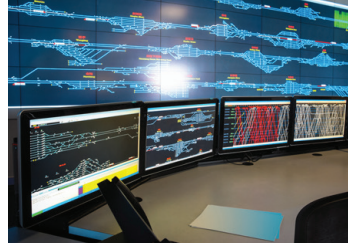
Train Control System
